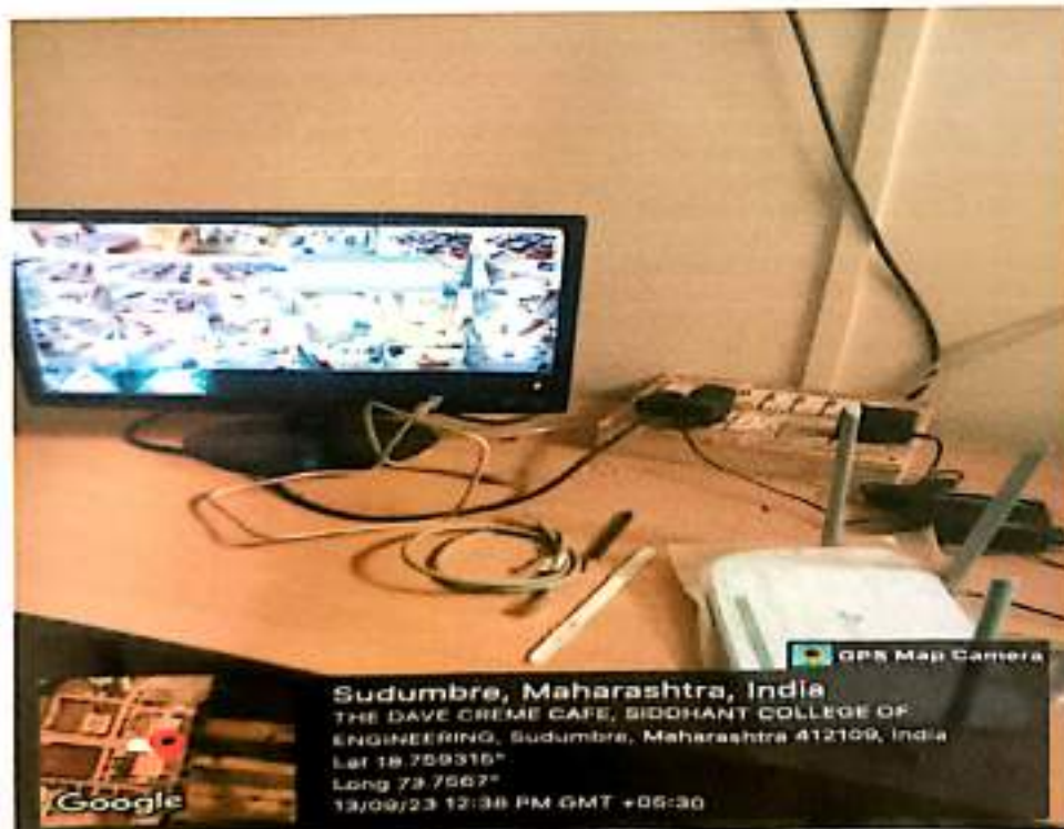
WIFI FACILITY AND CCTV DISPLAY
