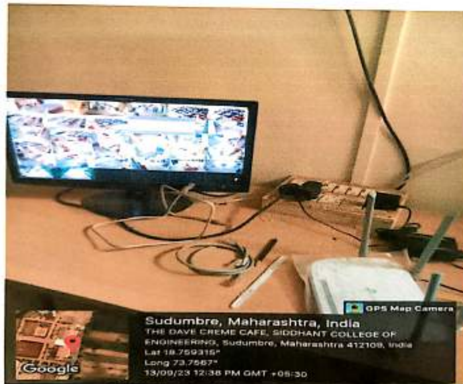
WIFI FACILITY AND CCTV DISPLAY
