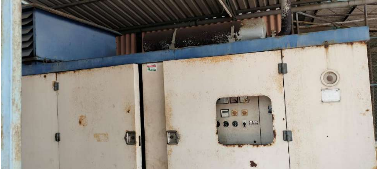
Photo-4: DG set up at Siddhant College of Engineering, campus Pune
