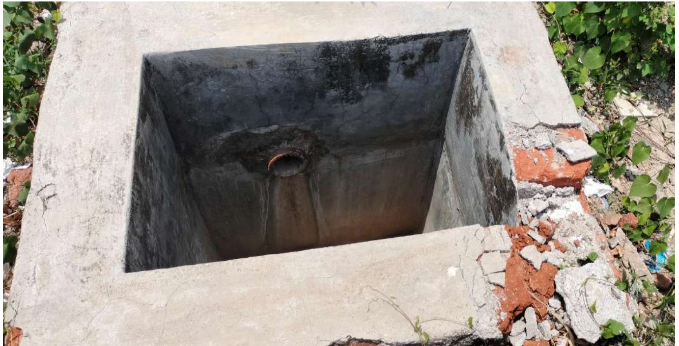
Photo-6: View rain water collection from building
