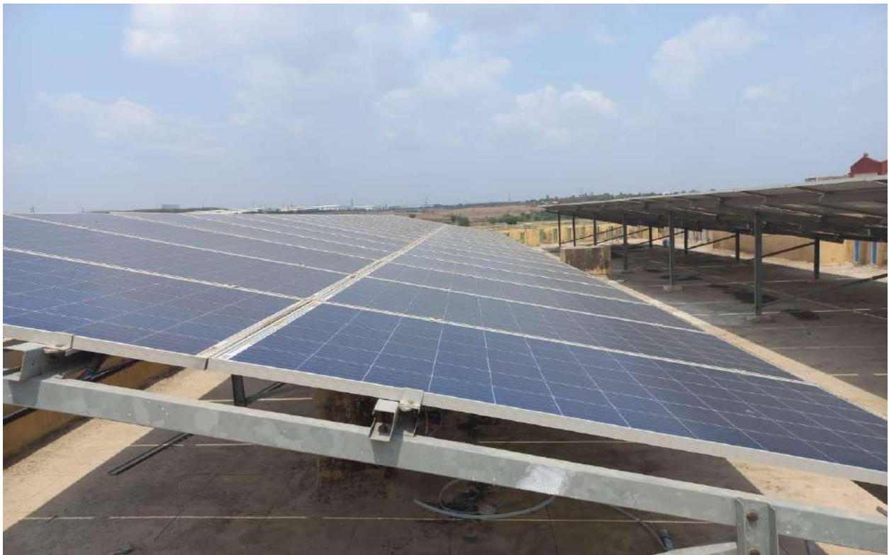
Photo-2: 221 kW solar roof top on Siddhant School building roof.
